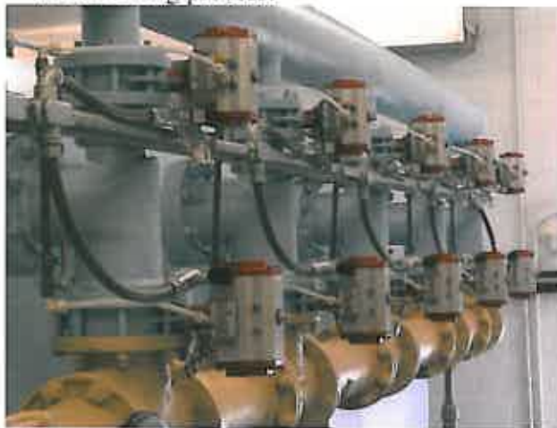
Air Powered Actuators on the Well 3 Iron Removal Filter
