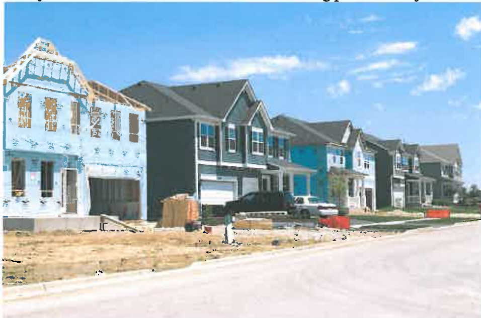
New home construction continues in the Liberty Lakes Subdivision in the Village of Wauconda
