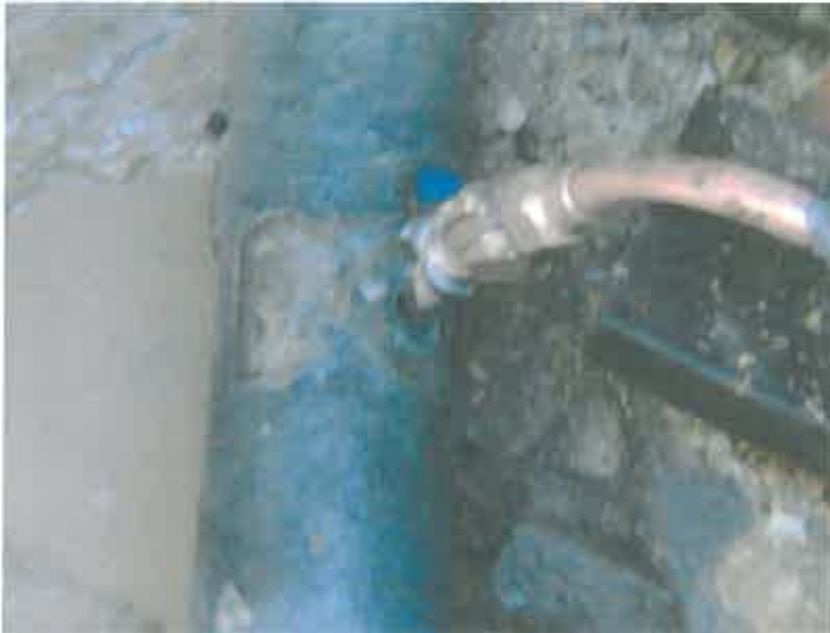
Broken Service Connection
